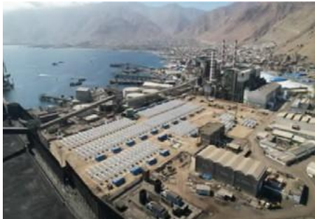
Tocopilla BESS (116 MW)
