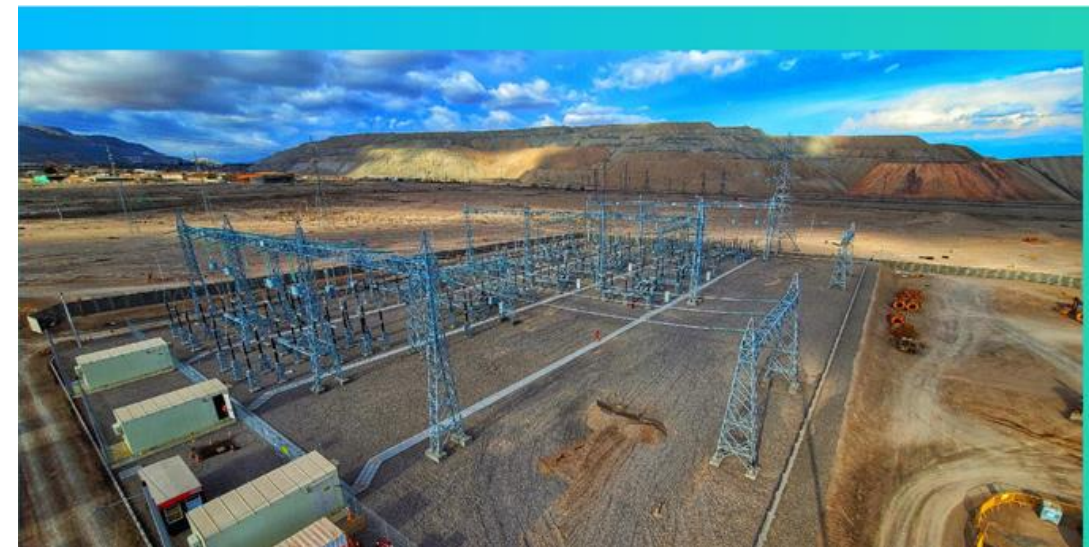
Nueva Chuquicamata (National) Substation + 2 x 220 kV transmission line Project completed / CEN recognition 06-Dec-2021
