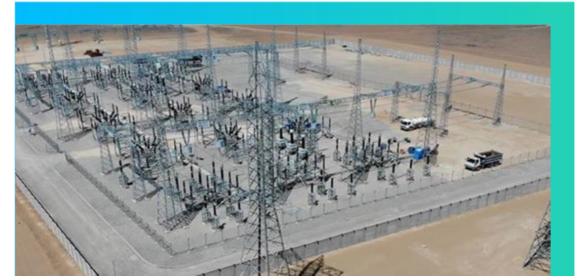
Algarrobal (National) 220 kV sectioning substation Energization: July-21 / Commissioning: Aug-21
