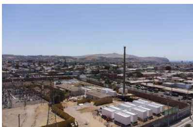
30MW BESS Arica * US$50 million CAPEX COD(e): 2H 2026
